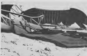
PARTIALLY DISMANTLED spherical gives the impression of half-eaten, metallic tangerine. High corrosion, as well as many years of service, brought about their demise.
